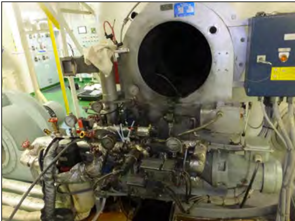
Figure 1: The damaged boiler
