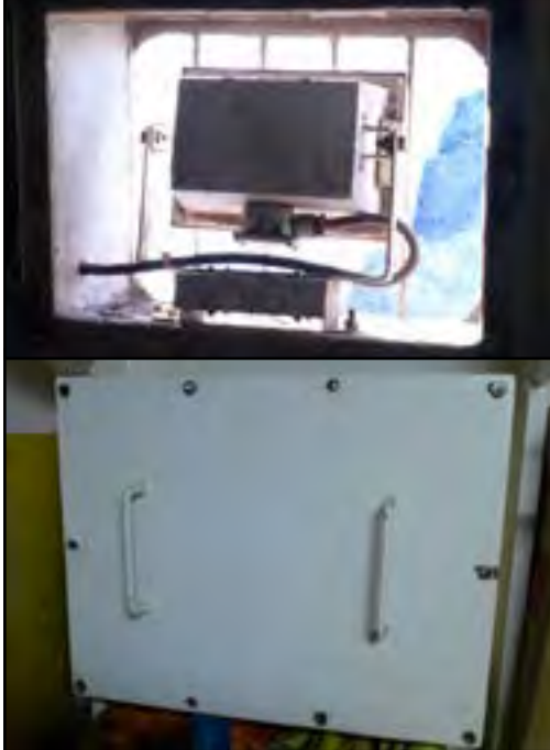
Cargo lamp access plate (removed and closed)
