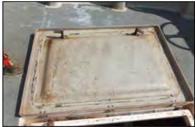
Figure 2: Missing hatch seal
