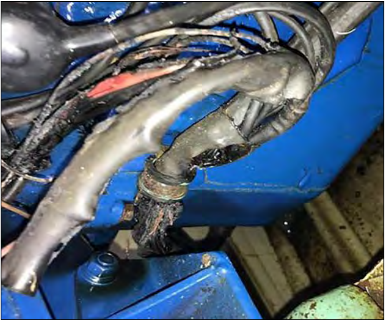
Figure 2: Heat damage to electrical cabling
