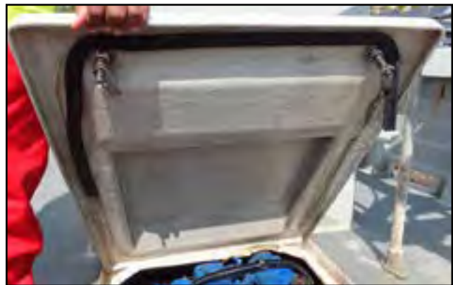
Figure 3: Damaged hatch seal
