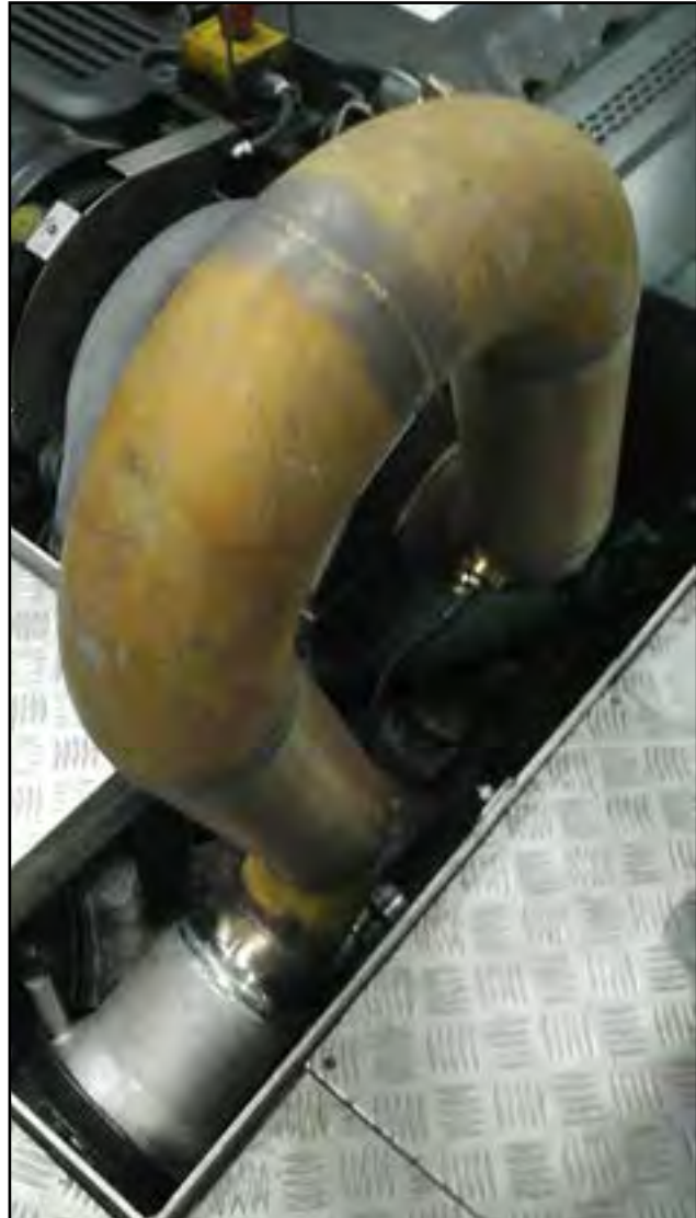
Figure: Starboard engine exposed exhaust pipe
